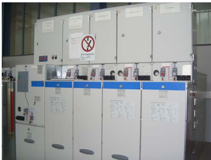
Fig. 27: Medium voltage switchgear of the LINS
