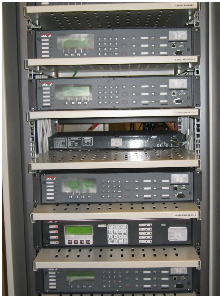
Figure 2-1: View of the rack with part of the equipments of the protection system
