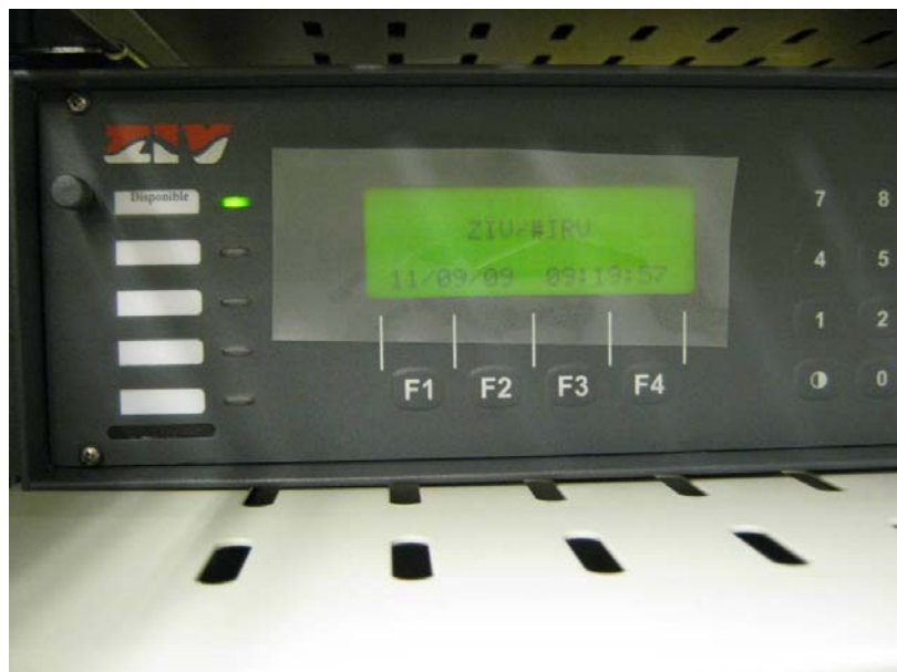
Figure 2-3: View of one of 8IRV installed in the demonstrator
