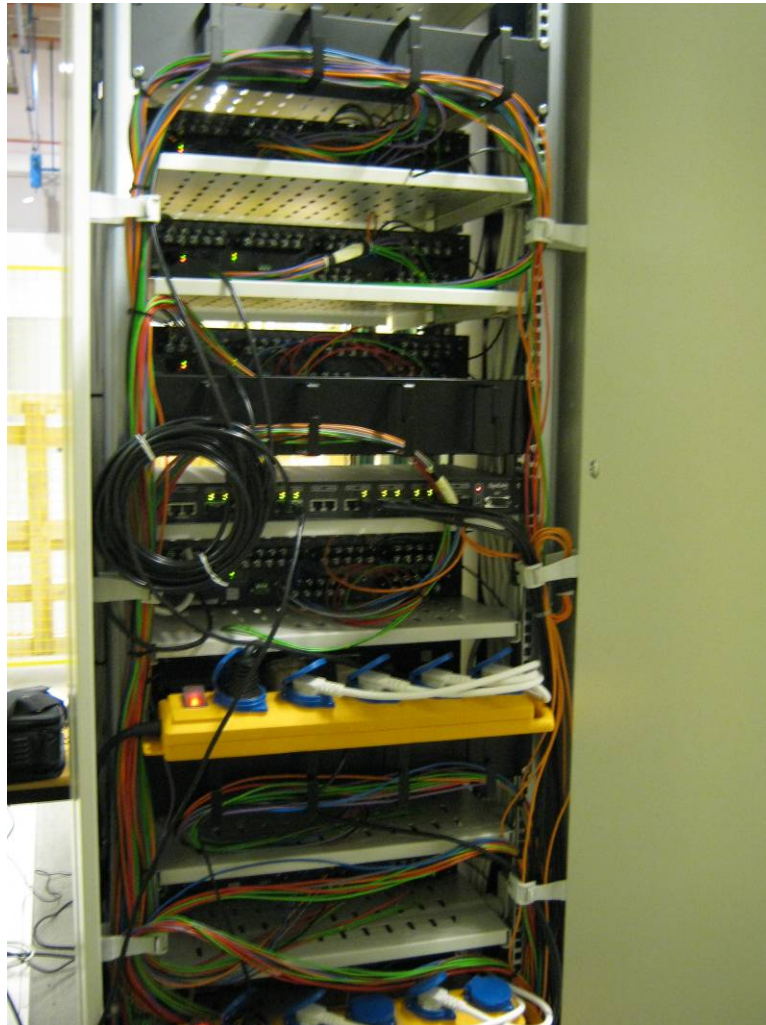
Figure 1-3: Back of rack with IEDs
