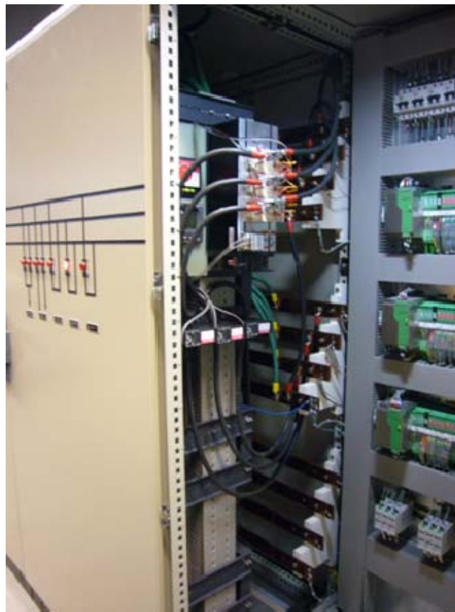
Figure 2-3: Deployment of the static switch inside the switching board
