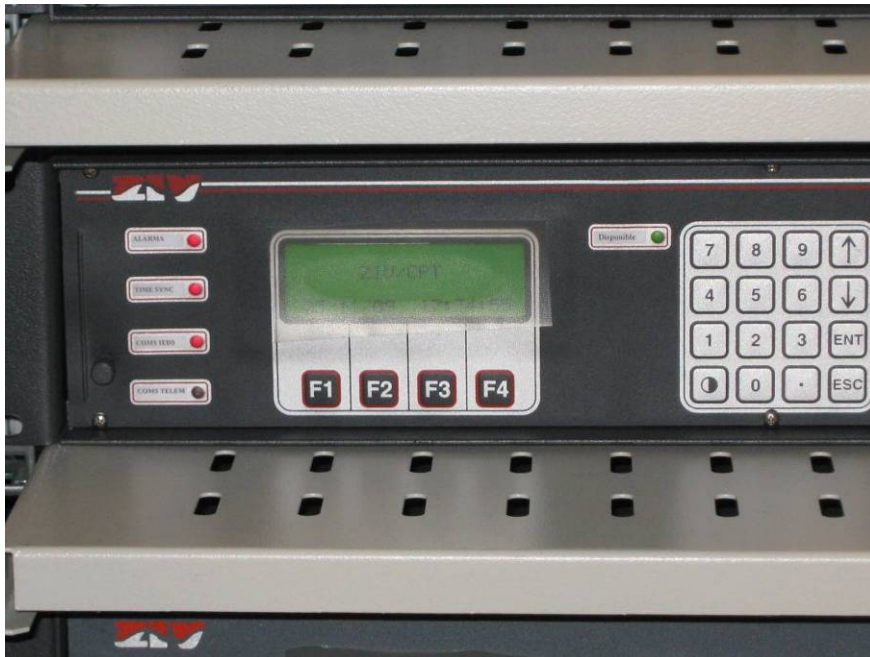
Figure 2-5: View of one of CPT installed in the demonstrator
