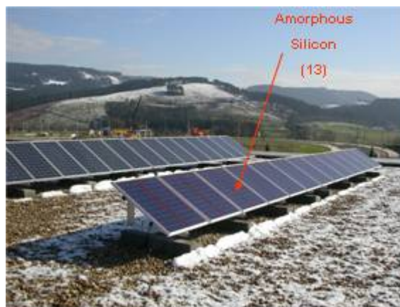
Figure 3-2: Amorphous structure based photovoltaic installation
