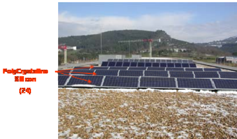
Figure 3-4: Multi-crystalline structure based photovoltaic installation
