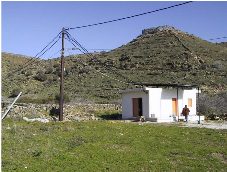
Figure 2: The “system hut” where the battery inverters, batteries, diesel generator and monitoring systems are kept.
