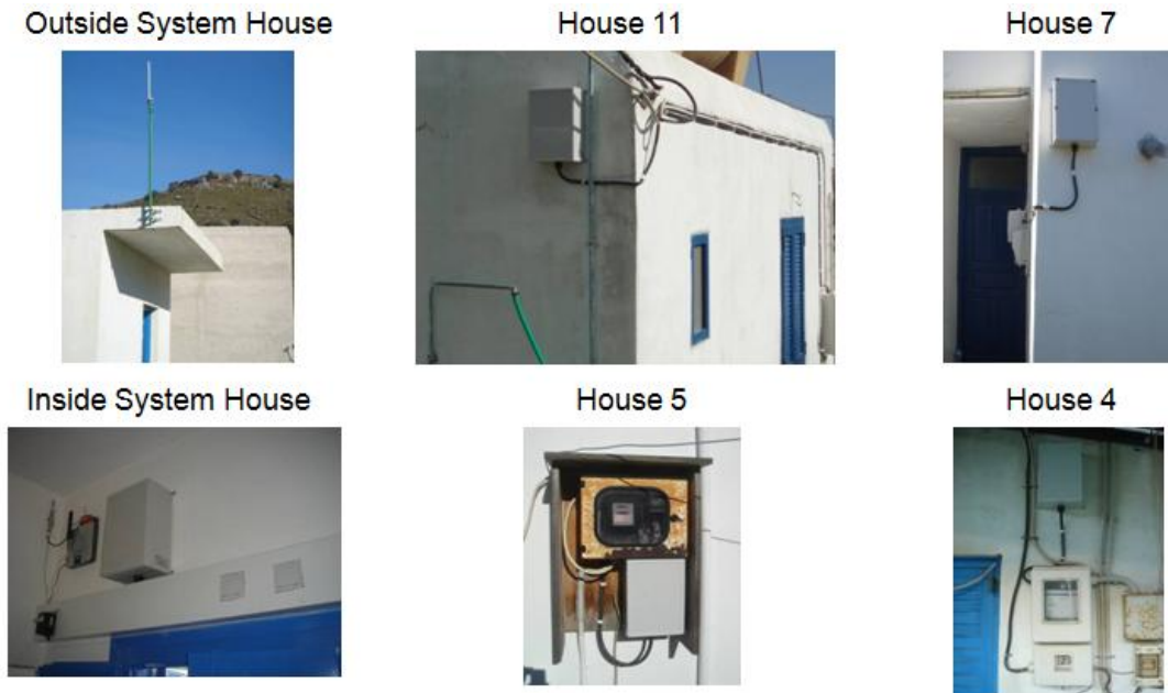
Fig. 2.3 The installed controllers
