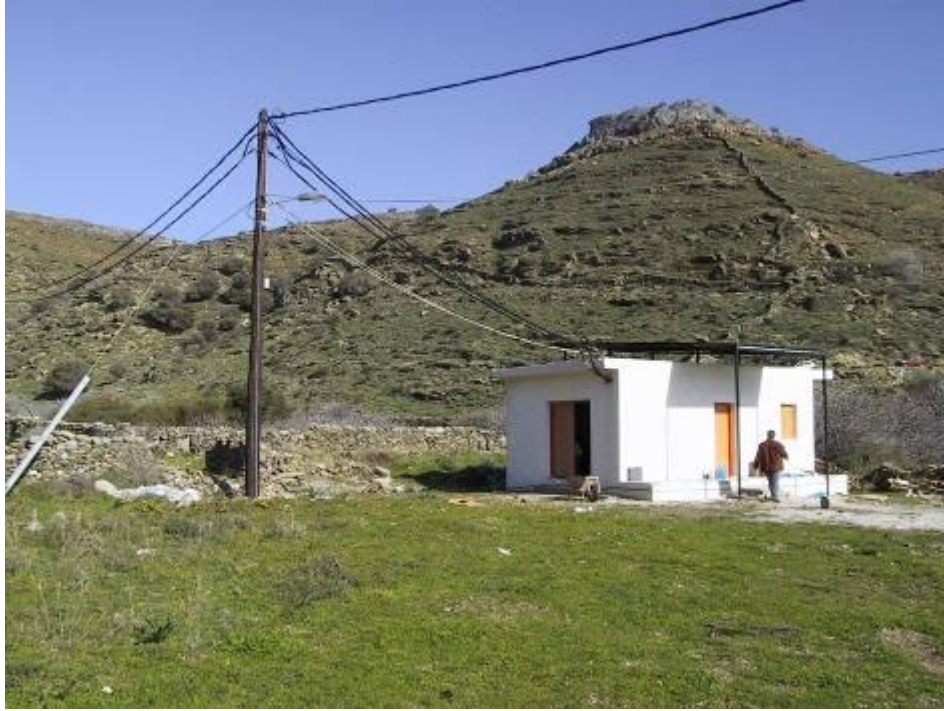
Figure 3: The “system hut or house” where the battery inverters, batteries, diesel generator and monitoring systems are kept.
