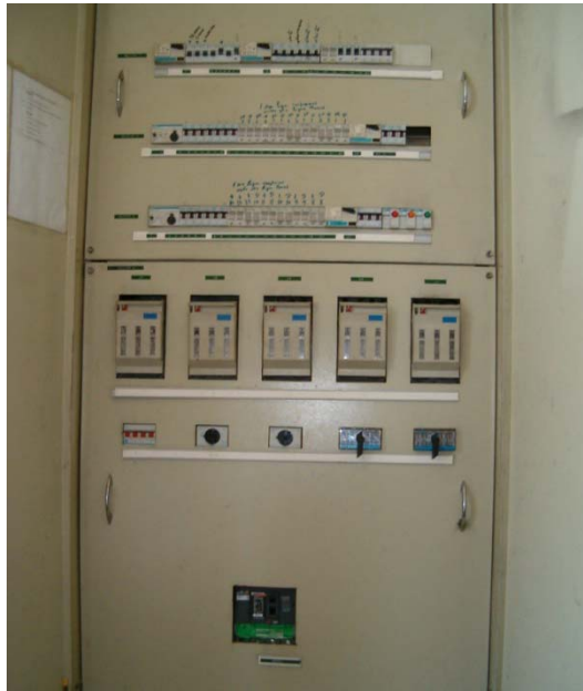
Figure 8 – Main switchboard of the Ílhavo MSP
