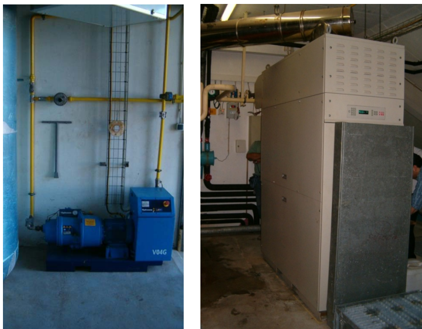
Figure 14 – Natural gas compressor (left) and Capstone 60 MicroTurbine (right)
