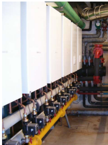
Figure 9 – Auxiliary water boiler, supplied by natural gas, and respective circulation pumps
