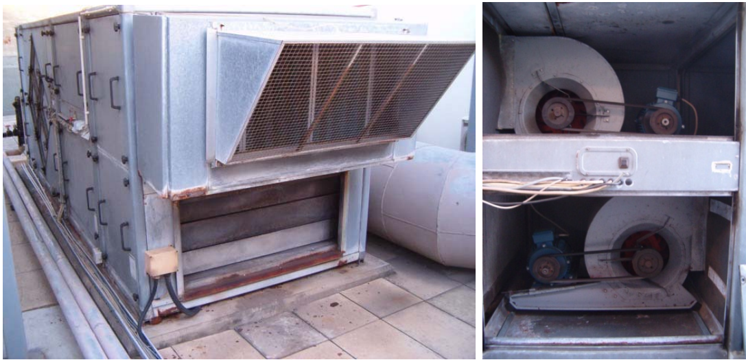
Figure 11 – ATU 3 and its respective extraction and blowing fans
