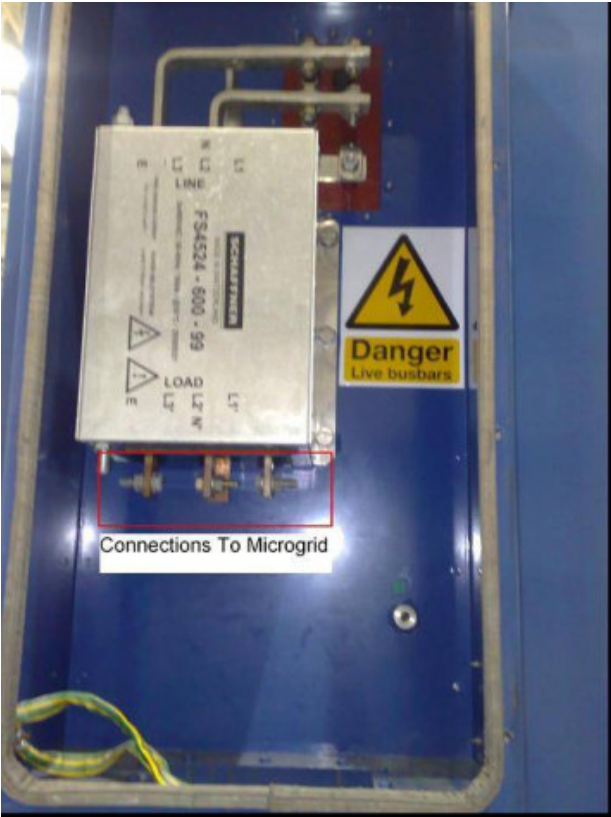
Figure 2.7 – Microgrid Connection (with Schaffner filter).
