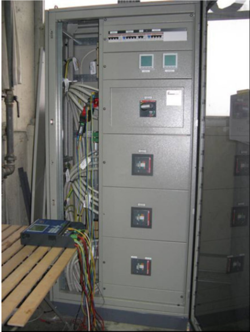
Figure 3.2 – Wally 1, installed on the I-Power Electric Board
