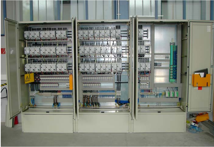
Fig. 34: Crossbar Switch Cabinet
