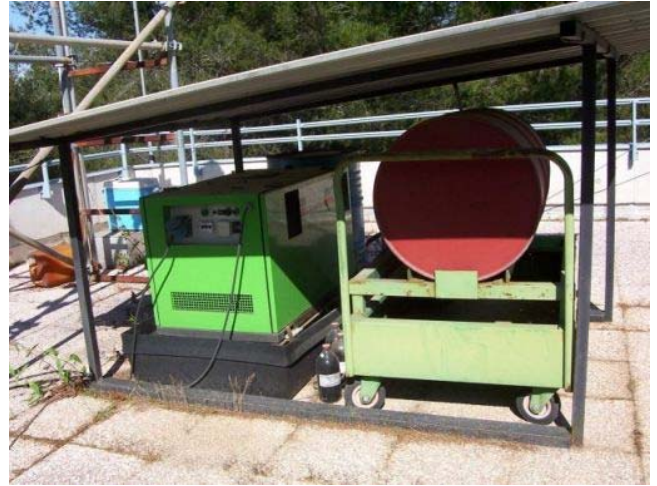
Figure 68: Diesel generator with its fuel tank
