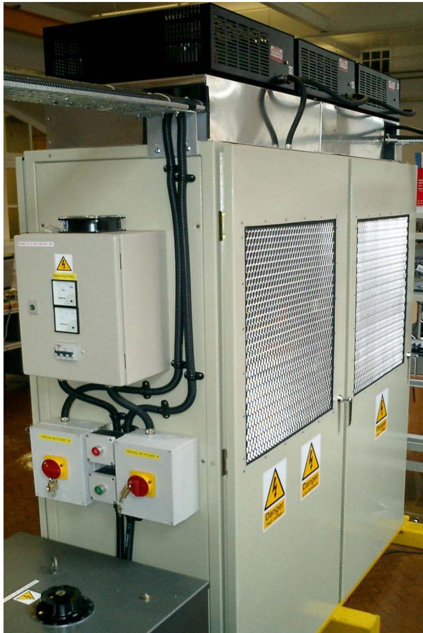
Fig. 60: Inverter/flywheel DC power source (inc. dump resistors)
