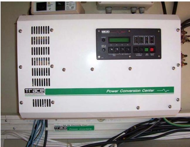
Figure 69: Trace SW4548E inverter
