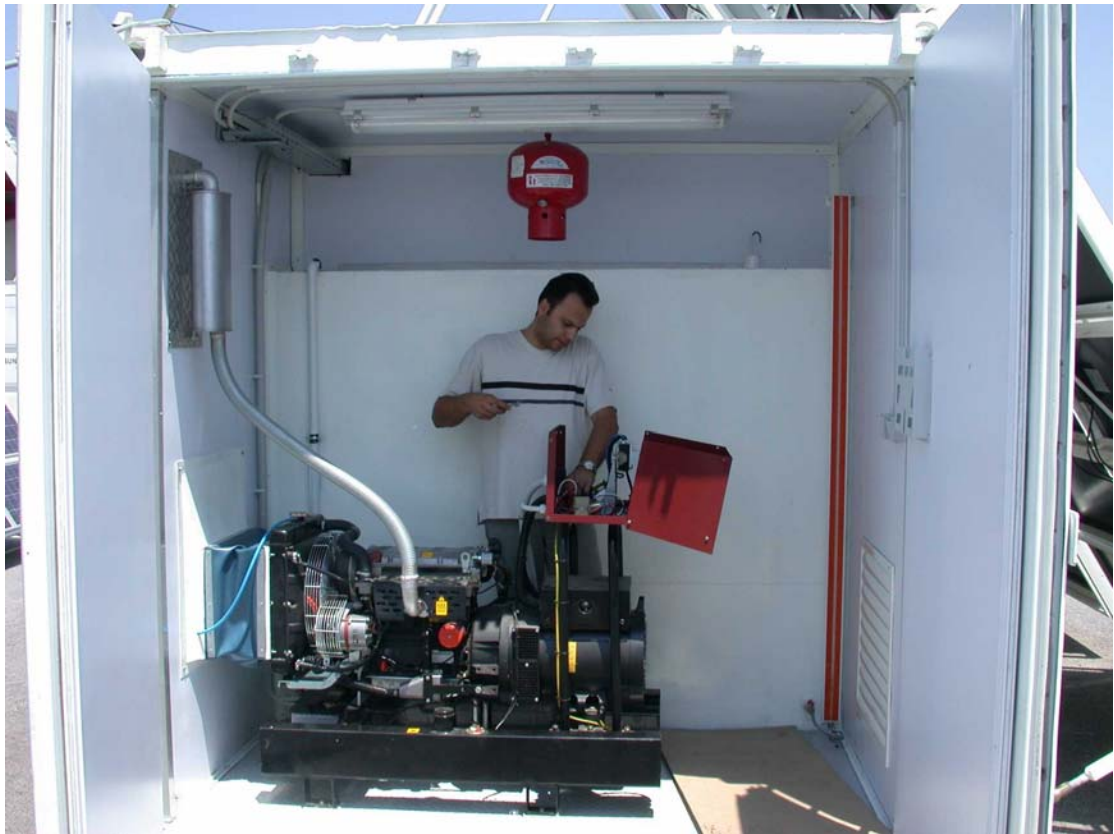
Fig. 48: A 10 kVA single-phase genset
