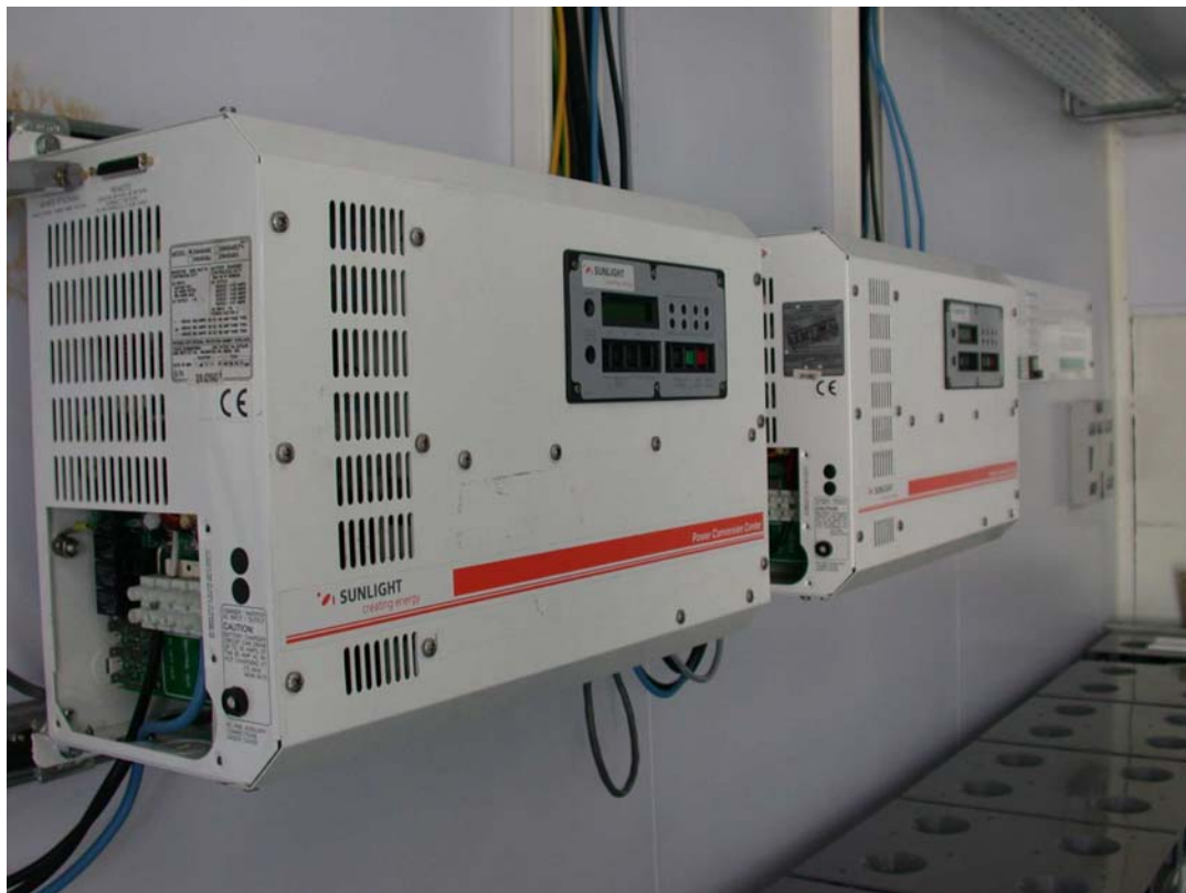
Fig. 46: Single phase inverter-charger consisted from two parallel single phase inverters 4,5 kW each
