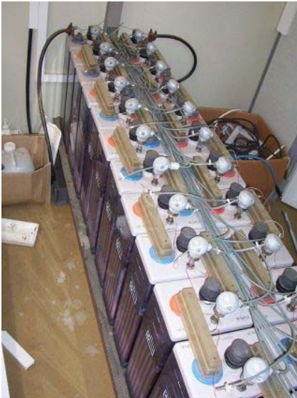
Figure 73: Battery with shunt resistors and temperature sensors
