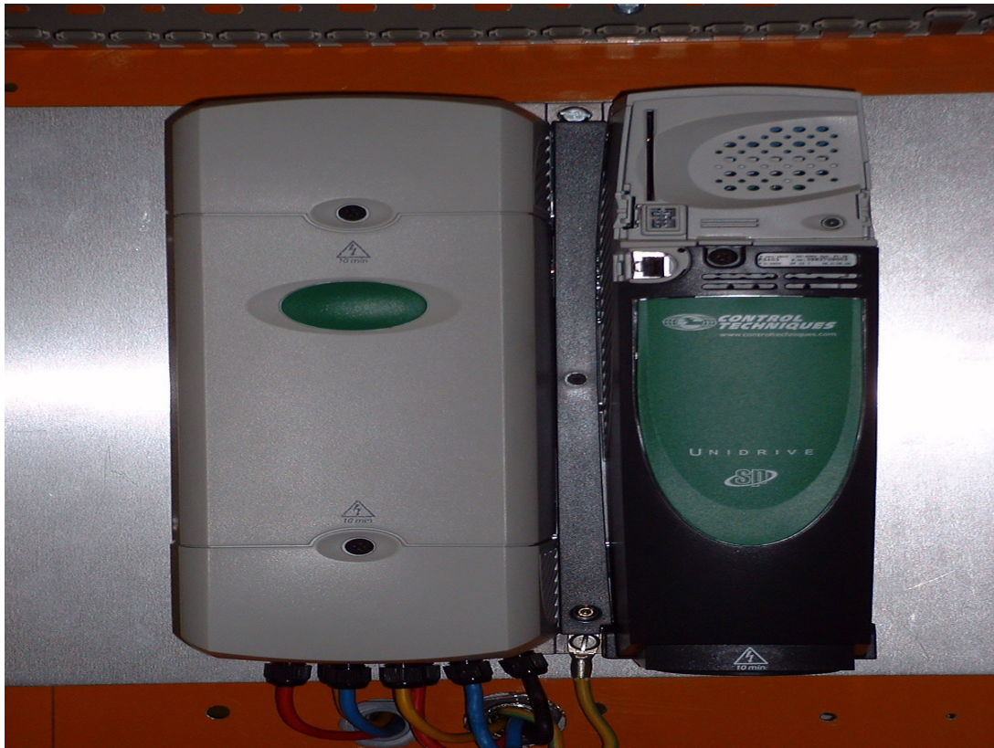
Fig. 58: 22kW AC motor drive
