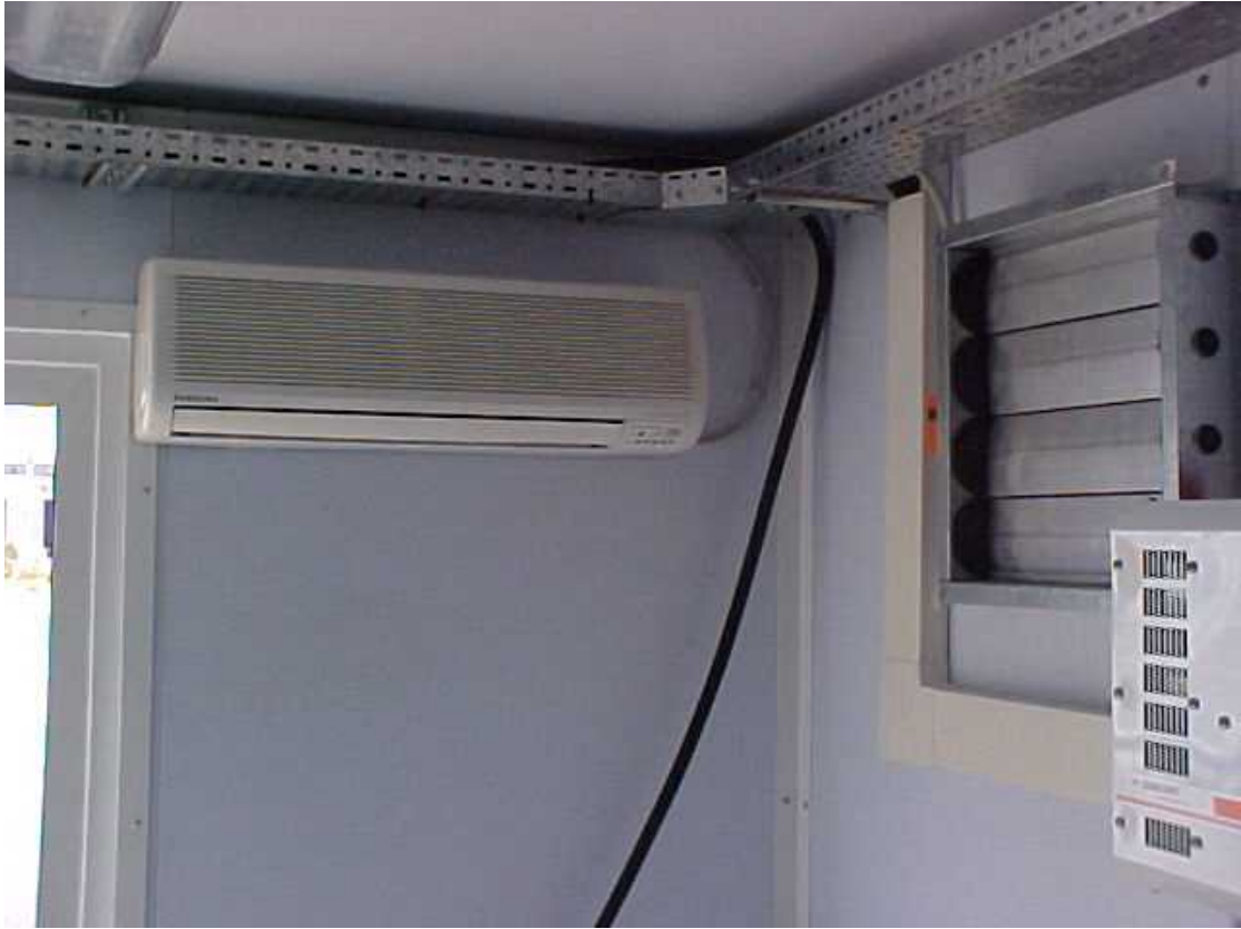
Fig. 47: A 2,5 kW Air condition unit, in the battery's chamber
