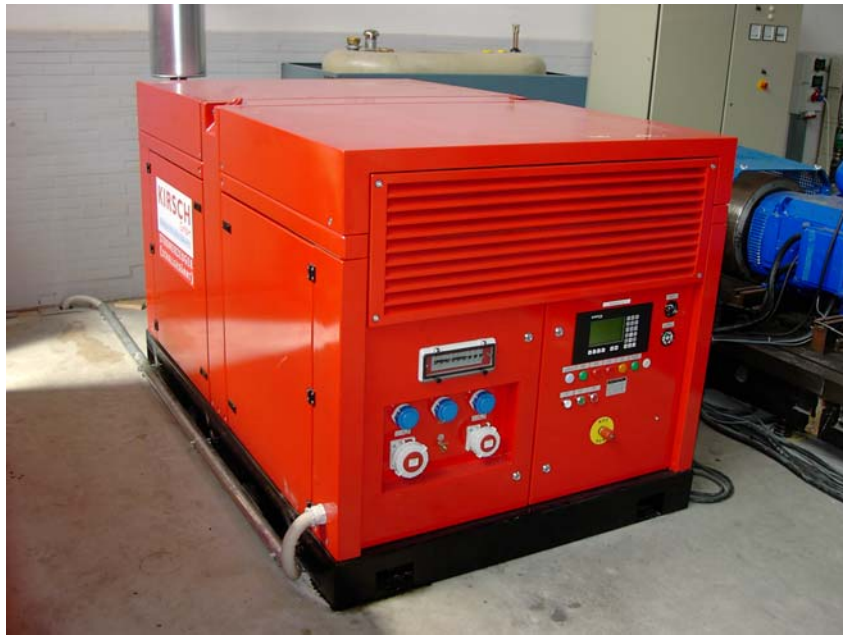
Fig. 14: Speed variable diesel aggregate
