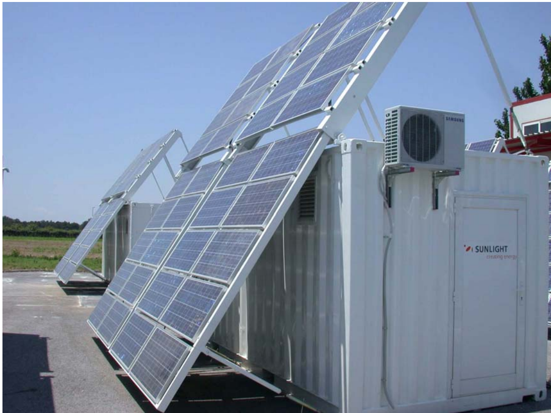
Fig. 43: Photovoltaic Panels (PV) of 3kW total peak output power
