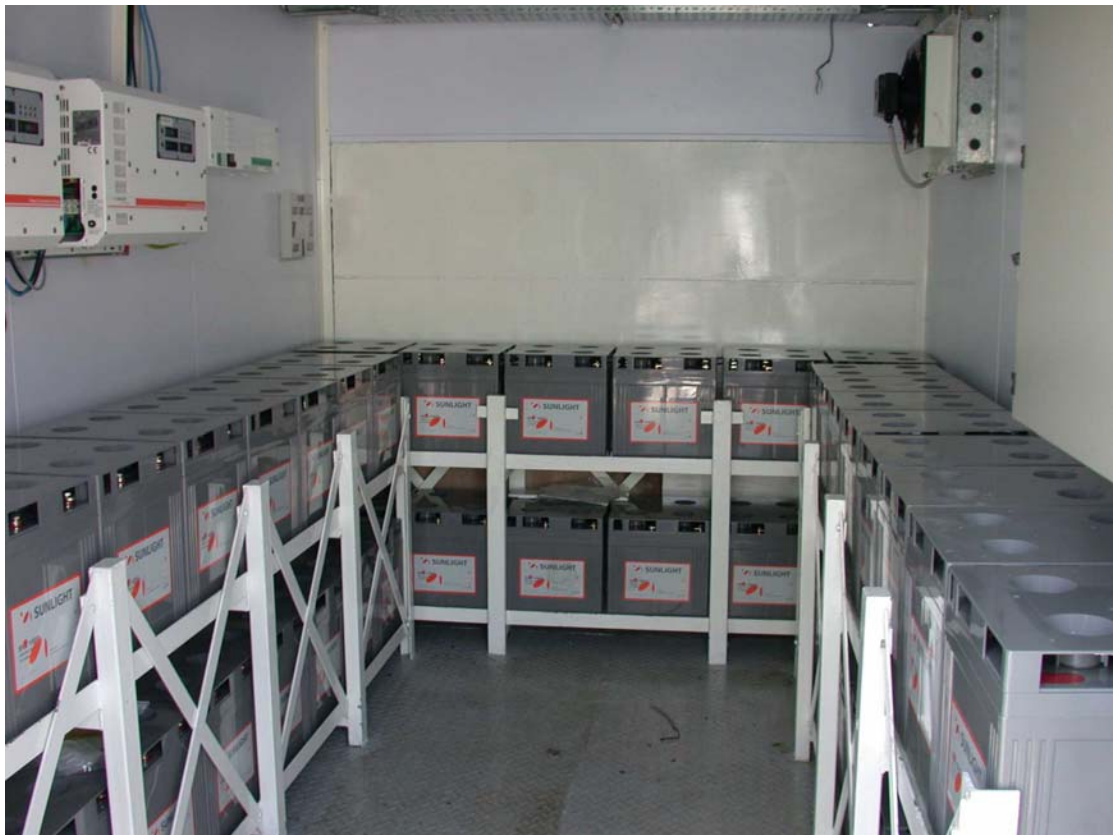
Fig. 44: VRLA Lead-Acid Battery string, 48V, 2 X 24 cells
