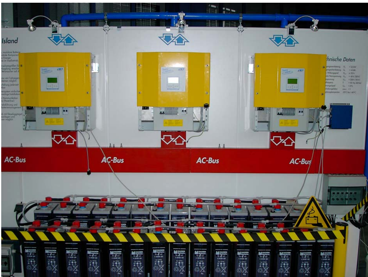
Fig. 39: "three phase cluster inverter" with RTU at the DeMoTec
