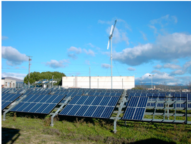
Fig. 5a: PV and WEC installation
