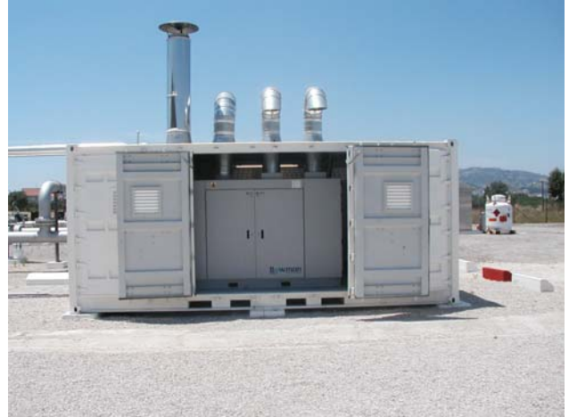
Fig. 3. Microturbine Bowman installed in the NG Station
