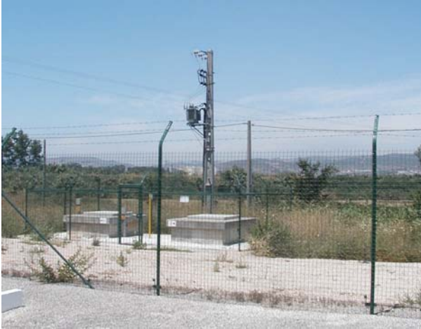
Fig. 2. Overhead MV/LV public distribution power station PTD 1063
